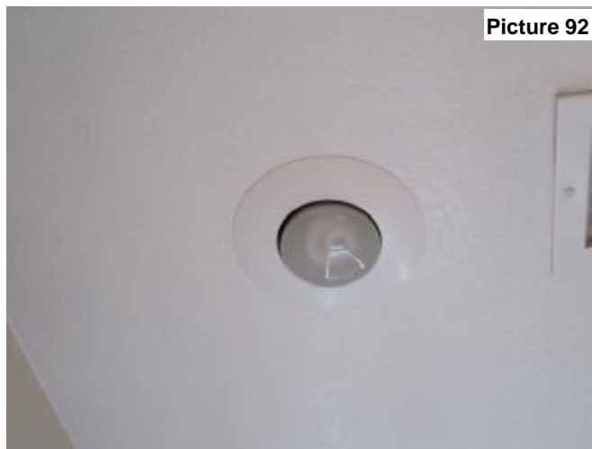
Light bulb in the upper left bathroom is burnt out.
