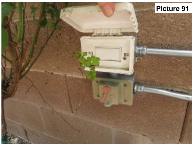
Light switch for the back yard block wall lighting.
