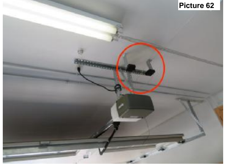
The single door automatic opener appeared operational.
