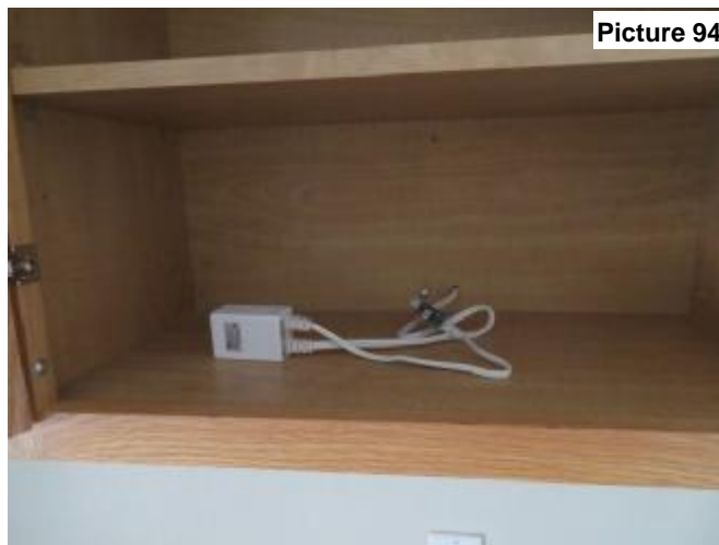
Upstairs desk area under the counter lighting is missing the lights.
