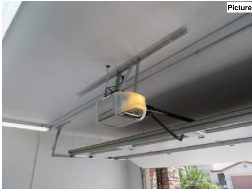
The double door automatic opener appeared operational.
